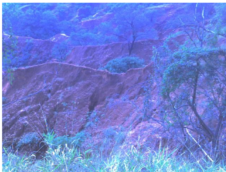
Figure 03. Voçoroca at Fazenda Santa Luzia. At the first plane, the limitation of the road whose drainage was converted to the plantation area.
